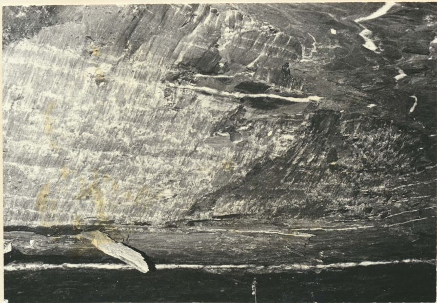
View of main slip-fracture in same roof fall as in previous photo. Clay dike runs along lower edge of the slip surface. The thin white band near the lower edge of the photo is the St. David Limestone.
