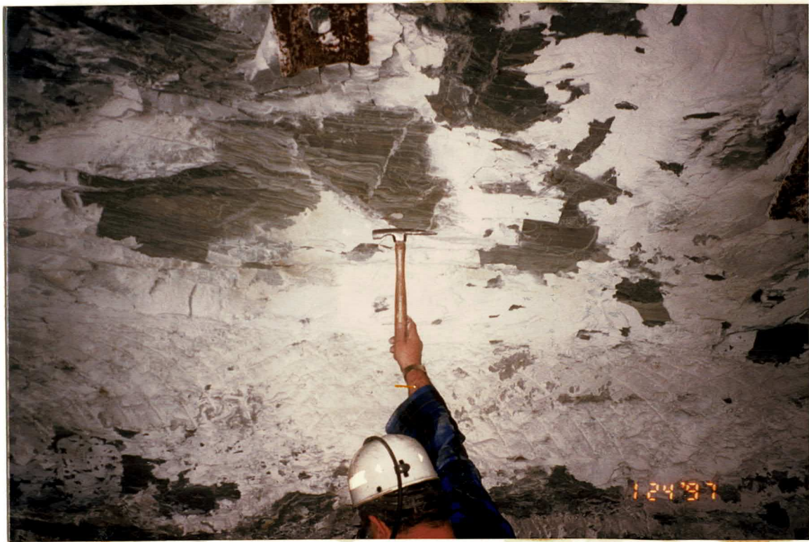
Location #5. Note sand-filled, near vertical fractures in roof sediments.
