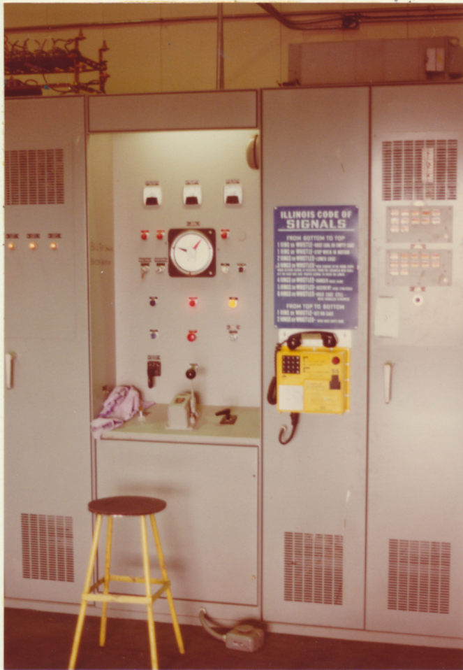
Control panel for hoist
