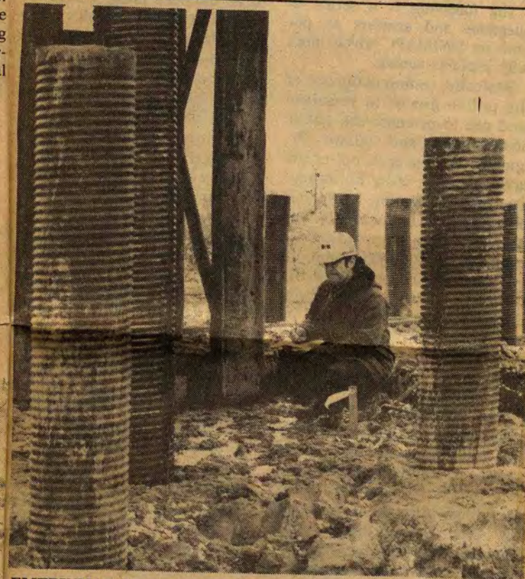
EMERY DIAL, Monterey employee, checking piling that will support coal storage silos.
