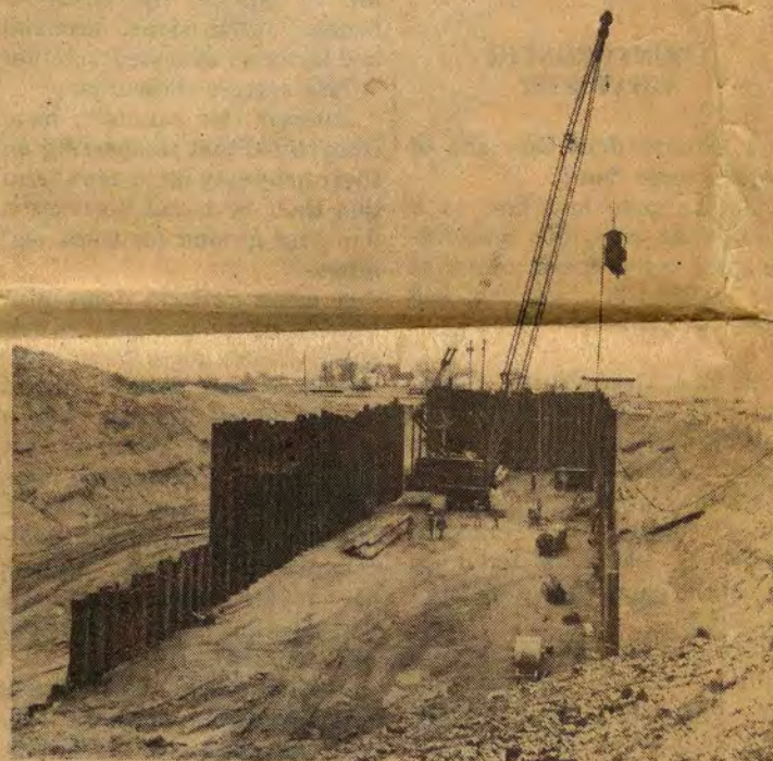
VIEW OF THE STEEL "COFFER" in which the upper portion of the slope will be constructed.
