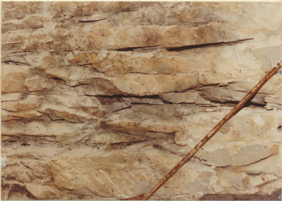
Location 3; open fractures in limestone roof. Roof bolt roughly 1 inch in diameter, for scale.
