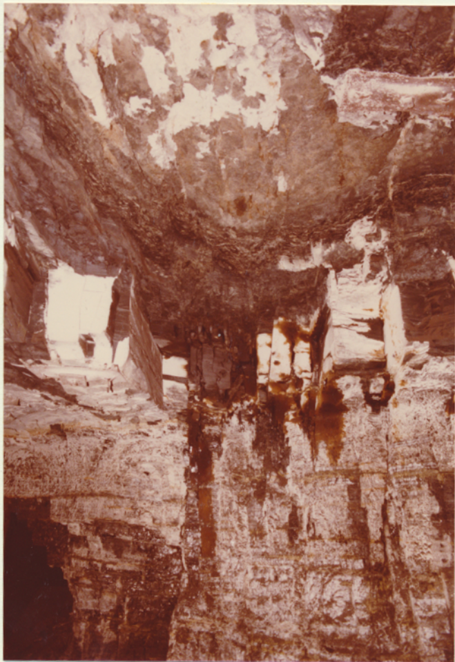
Oil-stained fractures along strike-slip fault in east entry of the 8th Main South. Top of entry is base of Brereton Limestone; black blocky Anna Shale below, then the coal. White color is rock dust.
