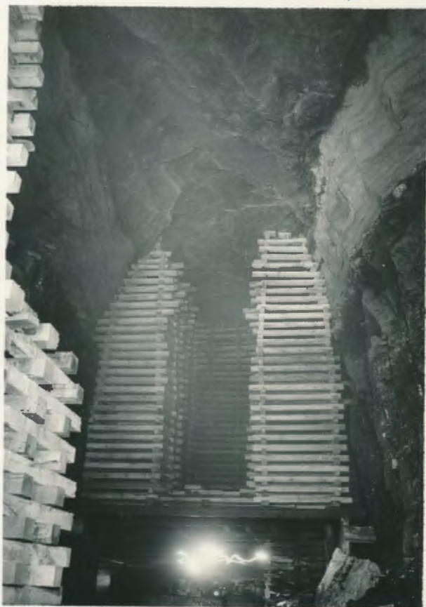
Massive cribbing in the 35-foot-high roof fall at the bottom of the syncline, where the coal is up to 13 feet thick.
